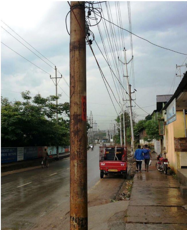
33 kV line inside city area of Assam
