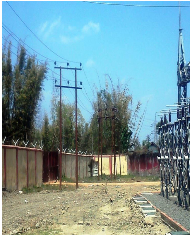
33 kV (H Pole) line inside substation
